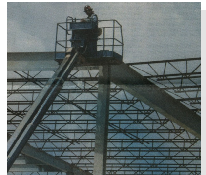
Construction of the Herrington Patriot Center, under way in August 2002. UT Tyler students could watch the progress broadcast live on the University website. {Ross Baker/The Patriot}
