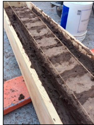
Figure 1. Construction of the wall foundation: Adobe bricks being placed in the wooden frame to form the footing.
