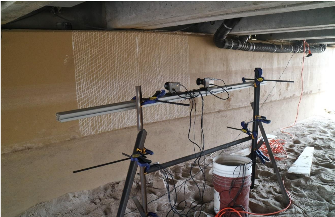
Figure 21. Hi-spec camera system for measurement of out-of-plane displacement of the bridge pier
