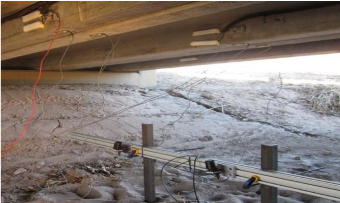
Figure 11. 2M System for monitoring an interior girder of UHPC span
