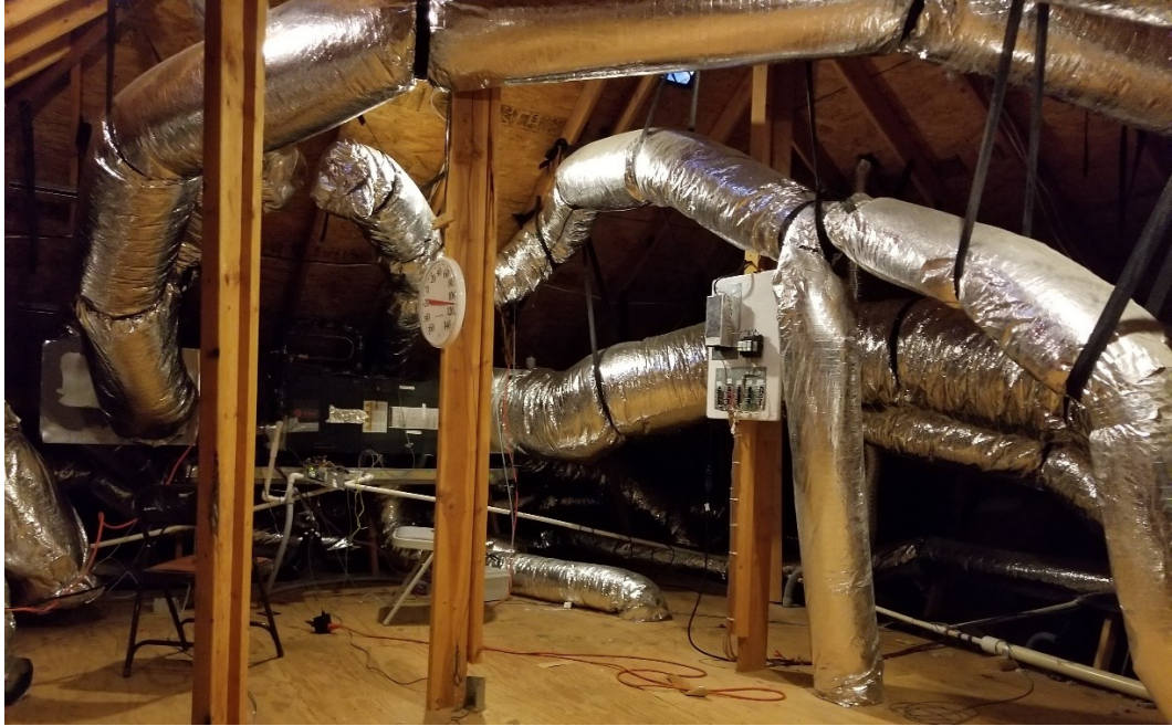
Figure 9. Air handler and ductwork in attic
