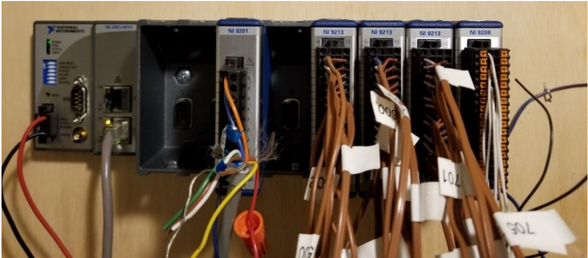
Figure C1. Used cRIO modules in NI-9074 chassis
