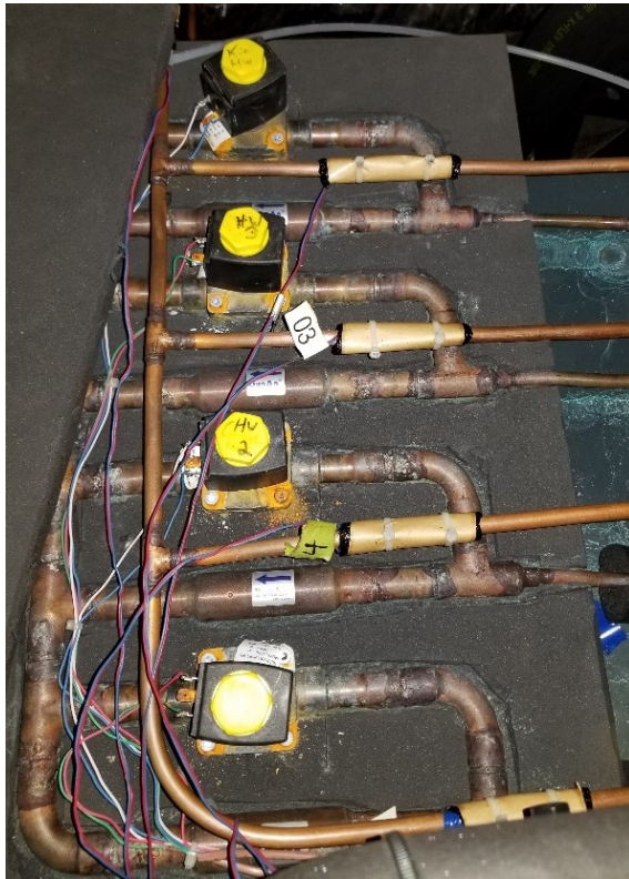
Figure 10. Refrigeration pipe manifold
