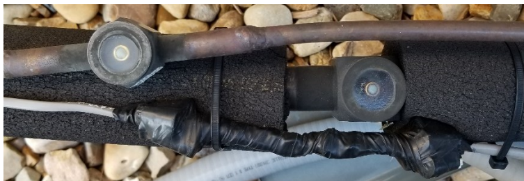
Figure 7. ODU refrigerant line sight glass
